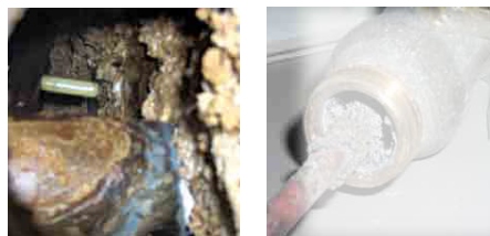
Hard-scale build-up on the plumbing system.
