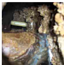
Hard-scale build-up on the plumbing system.
